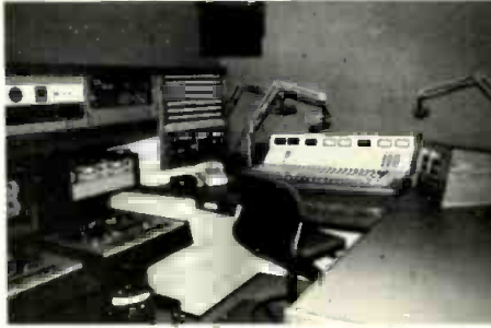
WDBO-AM's production studio is one of three production rooms in the new AM/FM facility.
