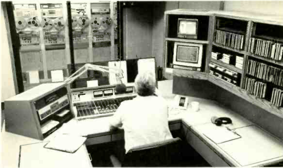
Announcer Bill Norris is able to look into the room, which holds equipment racks from KQXT-FM's on-air studio.
